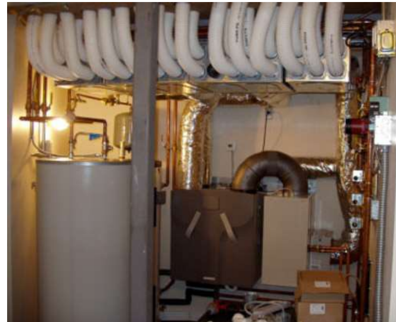
The ground source pre-heater or pre-cooler is the beige rectangular unit shown on the right of the HRV
